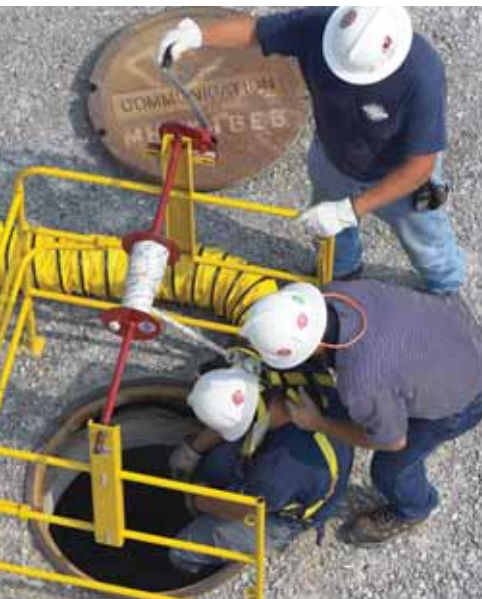
Service Electric combines classroom instruction with hands-on training like the confined space rescue drill shown here.
